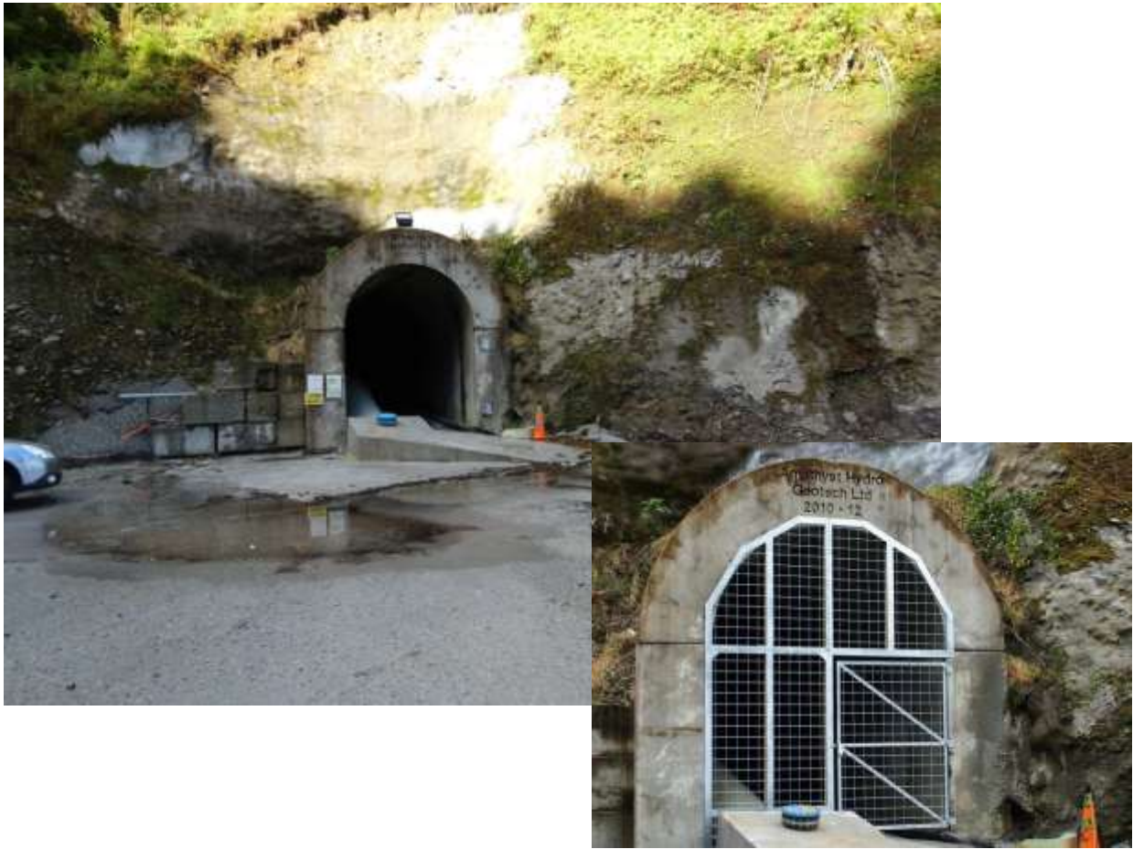
Figure 6: The Amethyst Portal – the penstock is buried on leaving the tunnel. (Note regeneration of vegetation above portal within 3 years).
